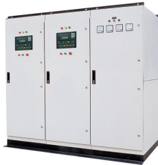
Parallel Control Panel system
